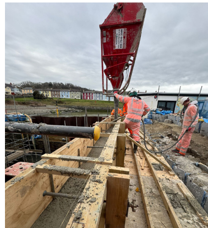
Pouring concrete via a crane to strengthen the HIVE rear wall garden
