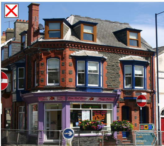
The windows surrounds are an inconsistent colour that do not match the shopfront
