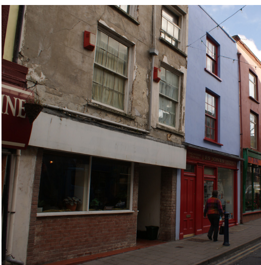
Evidence of a shopfront that has been unsympathetically altered in the past and poorly maintained
