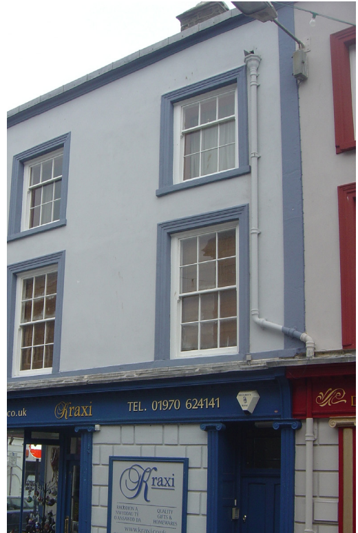
This downpipe is painted the same colour as the render to camouflage it
