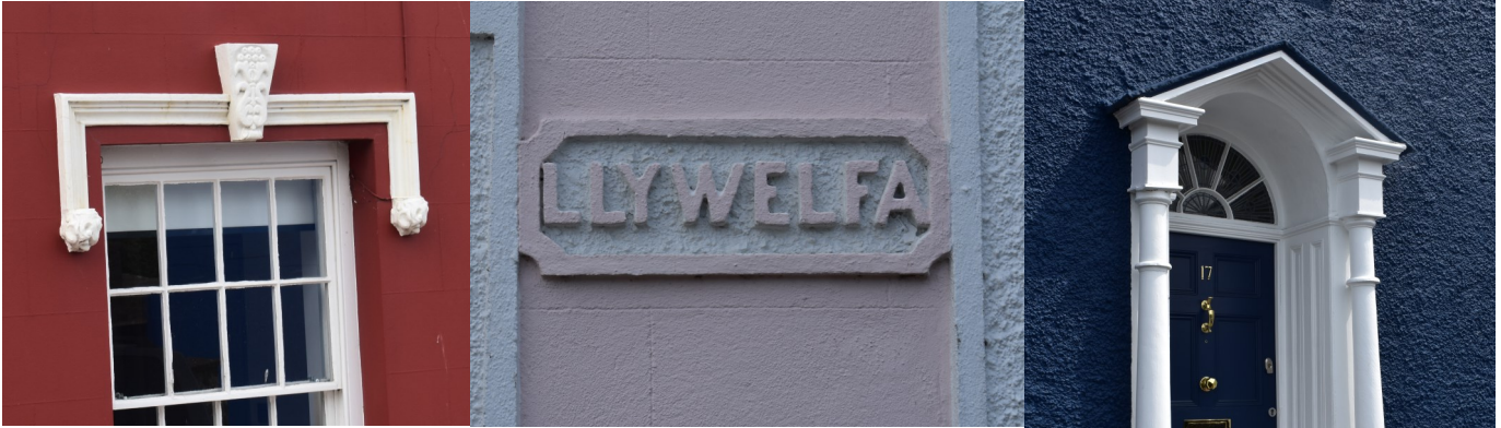
Figs. 17, 18 and 19 Hood moulding with decorative key stone, original house name plaque, and six panel door with fanlight, original stone steps and classical doorcase
