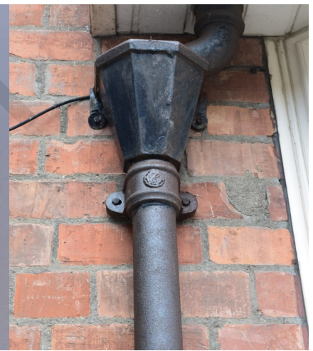
Fig. 29 Original iron hopper with high quality modern replacement downpipe
